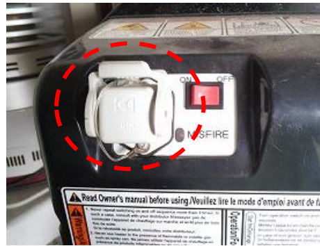
Picture 5 Inspection terminals for control device(PH1)
